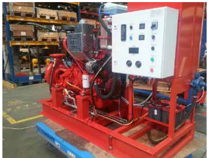
Customised Emergency Fire System
